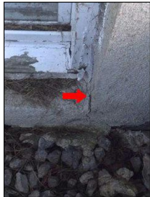
11. Typical minor cracks
