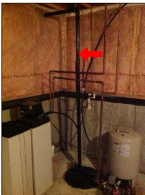
15. Missing check valve
