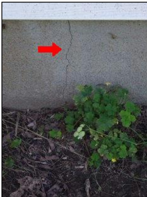
10. Typical minor cracks
