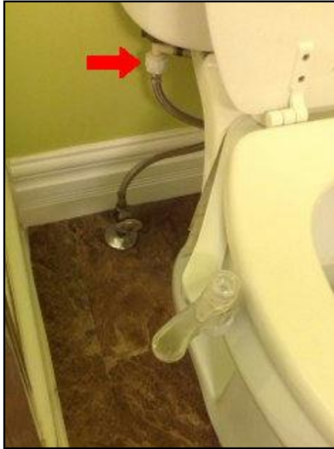
16. Backflow prevention missing
